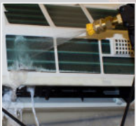
Clean coils from the front
