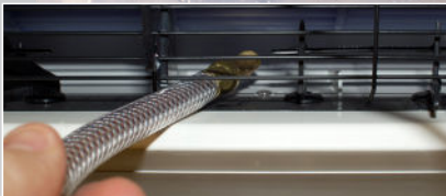
Clean inside the system
